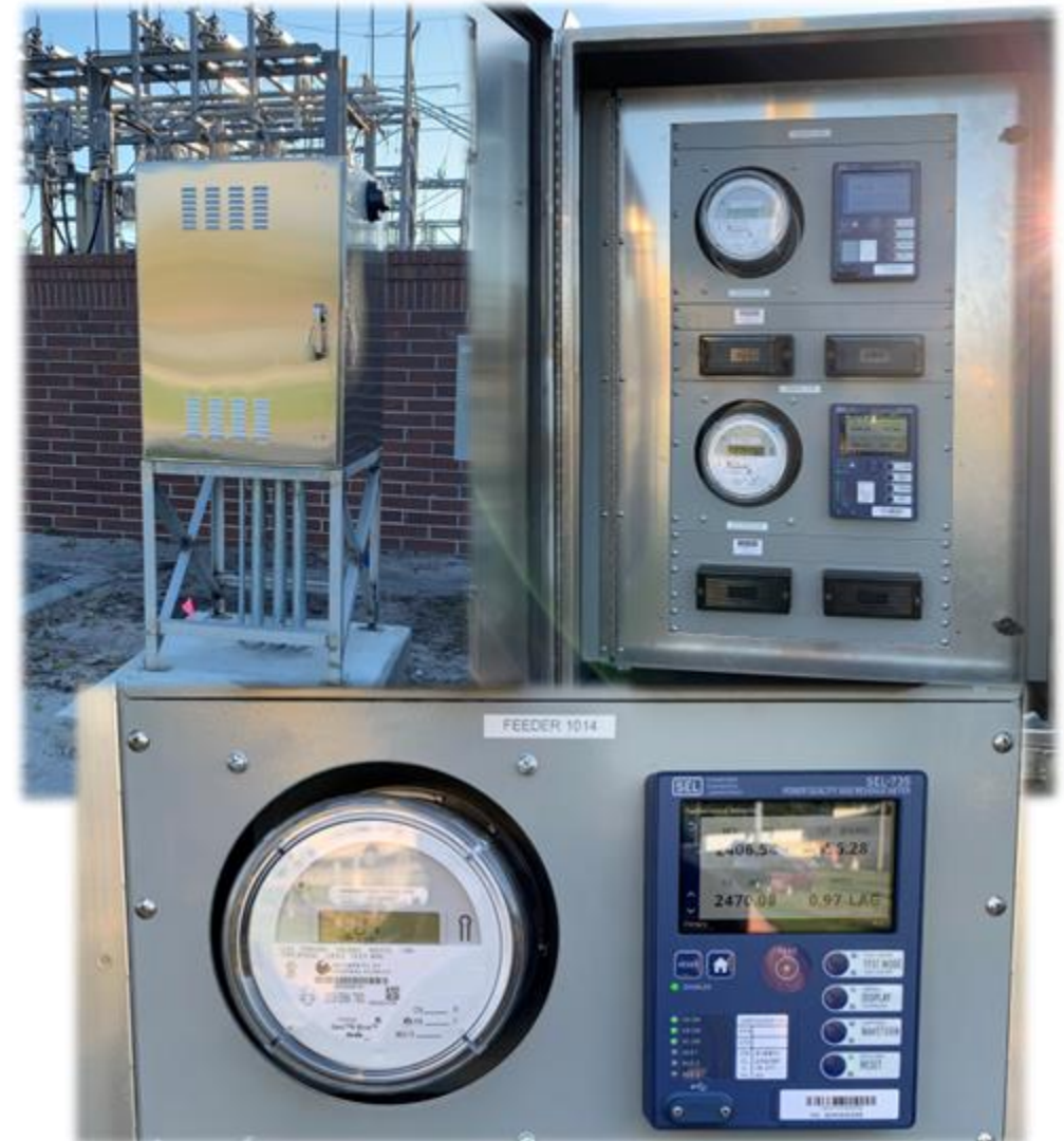
South Substation Metering for 2 Primary Feeders
