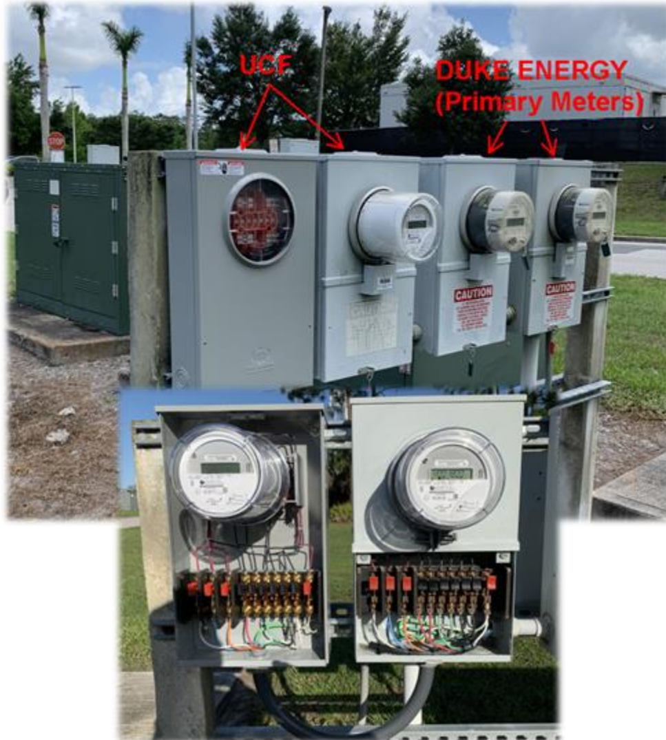
North Substation Metering for 1 Feeder
